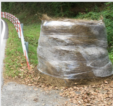
Guardrail nose not protected
