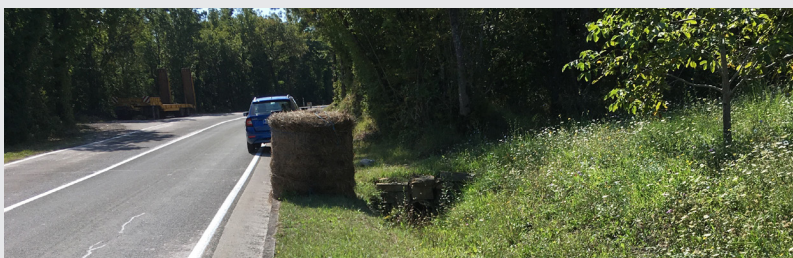
Concrete drain not protected
