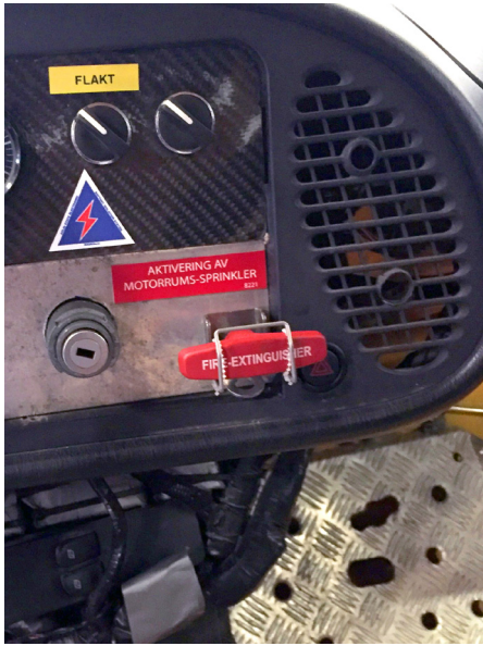
Figure 18. Installed activation handle with sign
