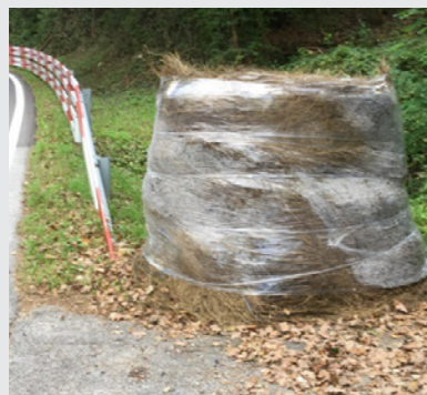
Guardrail nose not protected
