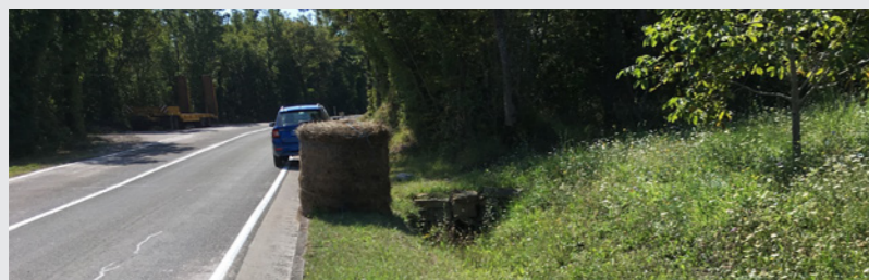
Concrete drain not protected
